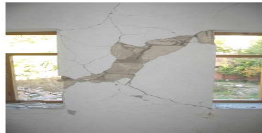
Figure 6. Damage between two wall openings
