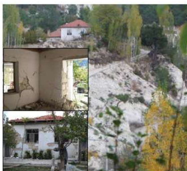
Figure 3. Damaged building due to slope
